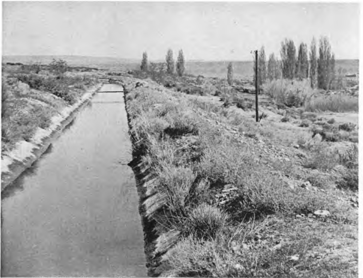
Trunk Irrigation Ditch serving the Richland Irrigation District. This ditch was partially concrete lined and in good condition at time of acquisition. This view was taken at the north edge of Richland.
